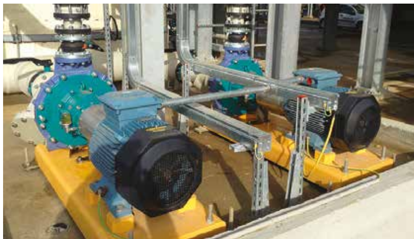
ITALY, Desalination plant
