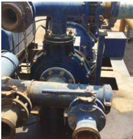
KUWAIT, Desalination plant Intake Pump. The very first Saturn
